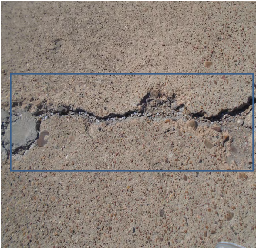
Crack between Product & Blending silos: Before
